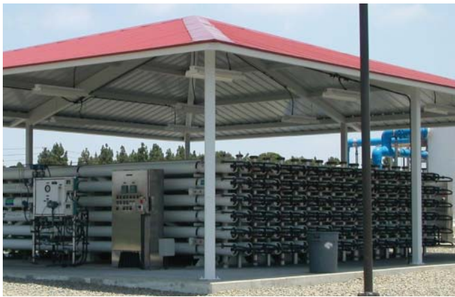
Figure 2. Reverse Osmosis Membranes at the Leo J. Vander Lans Water Treatment Facility, Long Beach, CA, Photo: Water Replenishment District of Southern California
