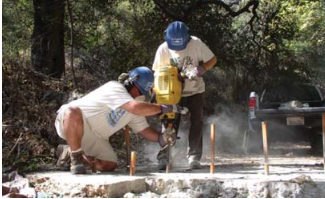
Figure 2. Drilling Holes with the Gas Powered Jackhammer and Placing Feathers and Wedges, Photo: Heal the Bay
