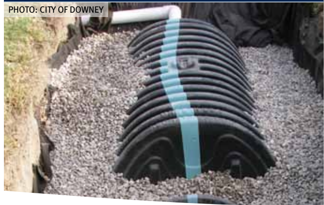
Figure 2. Residential Infiltration System at the Installation Midpoint
