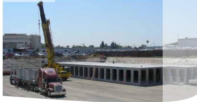
Figure 4. Regional Infiltrating Detention System Construction Under City (Discovery) Park PHOTO: CITY OF DOWNEY
