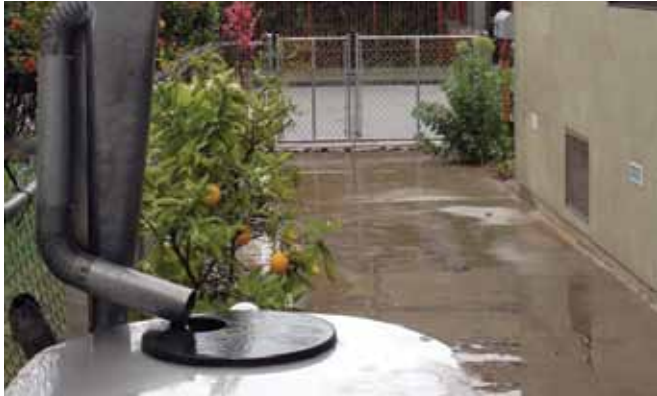
FIG. 10. The first-flush diverter collects the first rain and heavy matter to reduce pollutants in the cistern.
